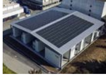
Figure: It is the largest production site in Dußlingen, where a photovoltaic system with a power of 110 kWp has been installed.
